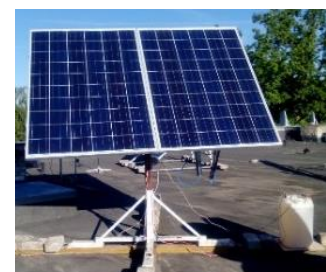
Figure 8. Dual axis sun tracker ST44M2V4P with two solar panels Solet P6.60-WF-250
