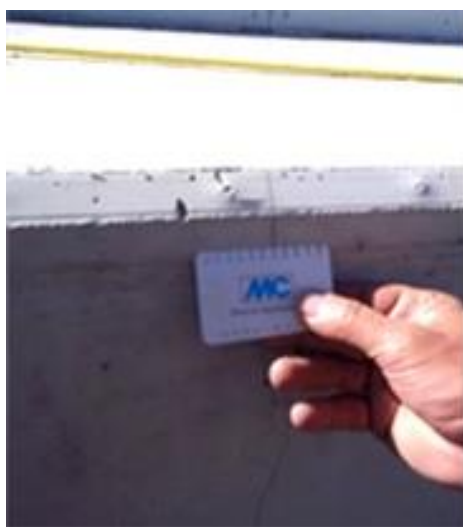
Figure 2. The illustration of crack width measurement using the crack width ruler
