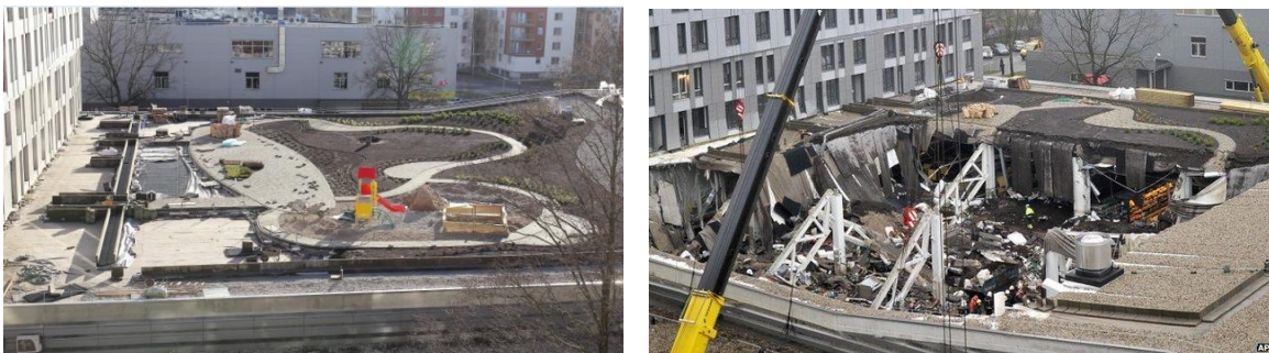
Figure 1. Maxima shopping center roof collapsed in Riga (before and after roof collapse). Photo by Gatis Smagars (Latvia...,2013)
